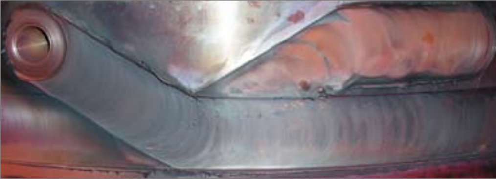
Figure 5. The start sequence and the exit hole above the joint line.
