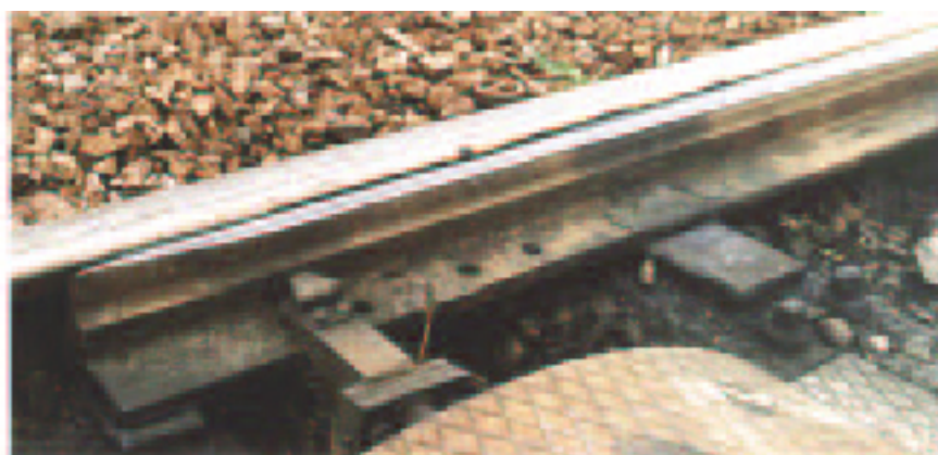
Figure 5. Worn and damaged switch blade.
