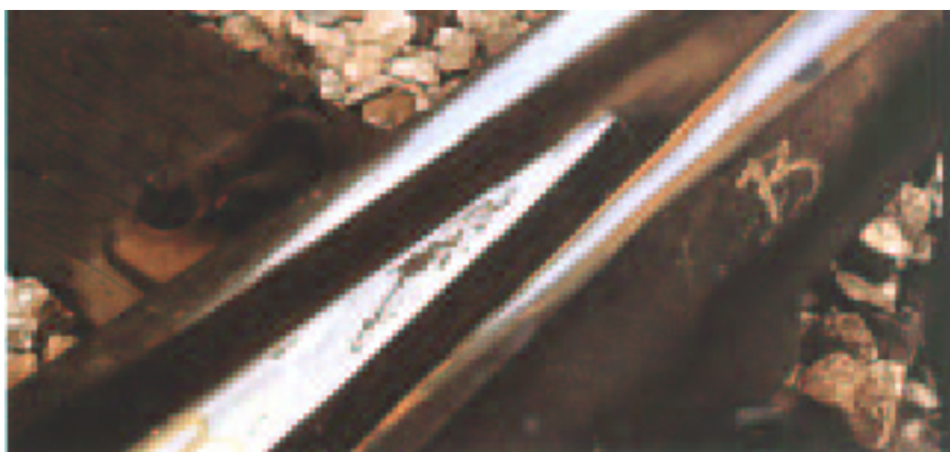
Figure 6. Cast defect in austenitic-manganese crossing.
