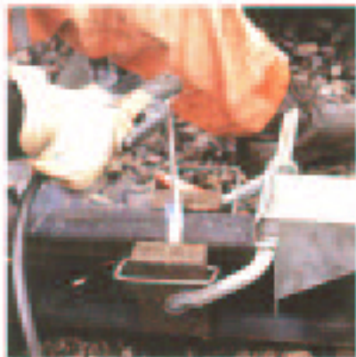
Figure 9. Coppershoes mounted for mould welding web and head with electrode OK 74.78. OK 83.28 is used for the cap layer.
